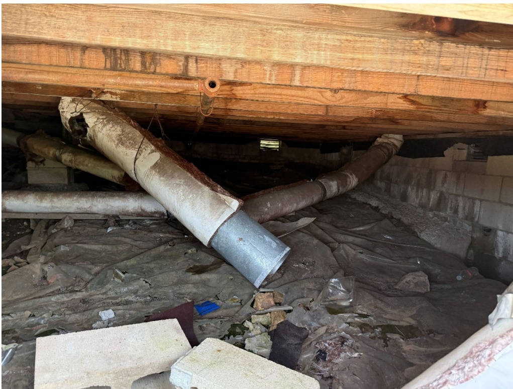
Photograph 4: A view of the heating and cooling duct work under the floor of the house.
