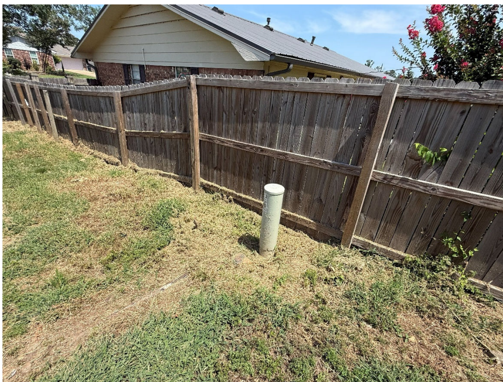
Photograph 4: A view of a connected utility equipment on the northern boundary.
