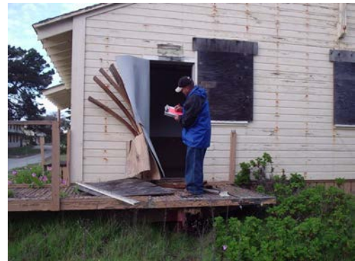
Strong enforcement measures help prevent demolition by neglect and ensuring that rehabilitation is completed in accordance with a COA.
