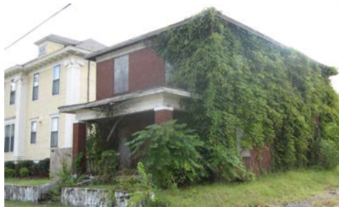
Abandoned dwelling in the MacArthur Park Historic District at 413 Daisy Bates.
