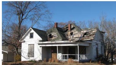
No overlay, no protection, no future. Without local ordinance districts or demolition-by-neglect provisions, this can be the result (4200 W. 16 th Street).
