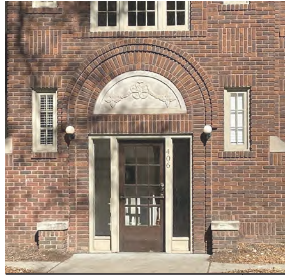
Repair deteriorated or missing mortar joints in masonry door surrounds to prevent water infiltration, 406 E 7th St.
