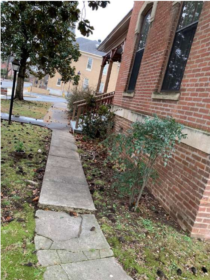
20. DAMAGED SIDEWALKS – NORTHEAST CORNER
