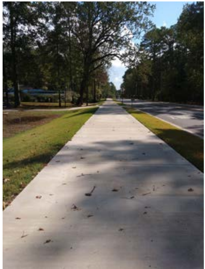
Figure 54: Recently installed sidepath just south of the new Little Rock Southwest High School on Mabelvale Pike. This was constructed by the City as part of the new high school construction and ancillary roadway improvements in this area. As new development or new roadway projects happen, these are key opportunities to continue filling in the paved shared trail network.
