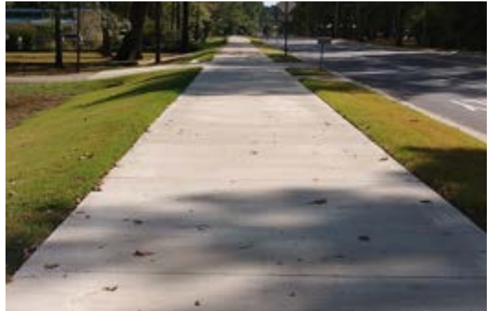
Figure 39: Recently installed sidepath just south of the new Little Rock Southwest High School on Mabelvale Pike. Away from Little Rock's urban core, sidepaths are an important facility for achieving roadway separation in the suburban Little Rock context.
