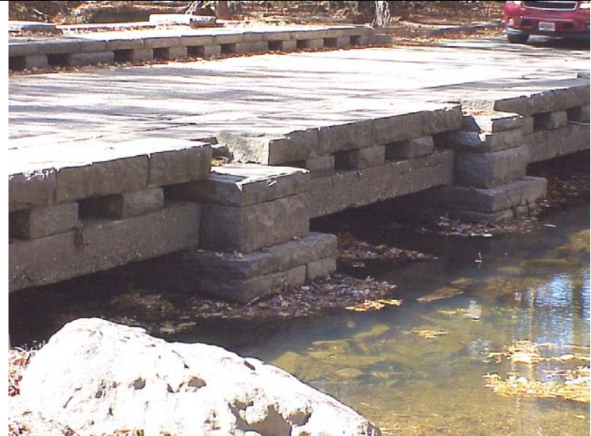
Piers on north side of the low water bridge over Rock Creek.
